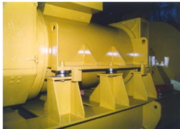
Figure 2. A Generator on Vibracon ® SM Elements.
