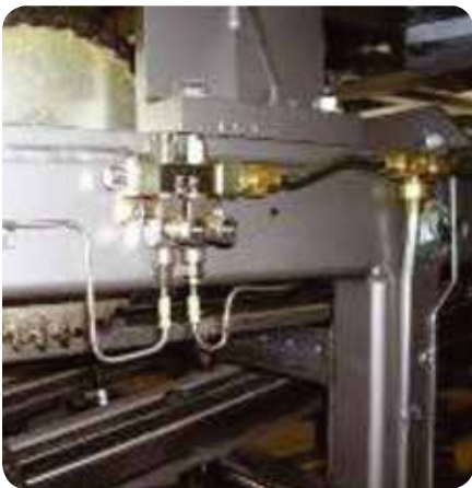
Stainless steel SL-32 grease injectors are used here to prevent corrosion from daily wash-down maintenance practices at this food plant.
