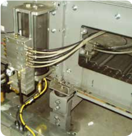
An Orsco VSR system lubricates a conveyor chain on an oven application in a food plant.
