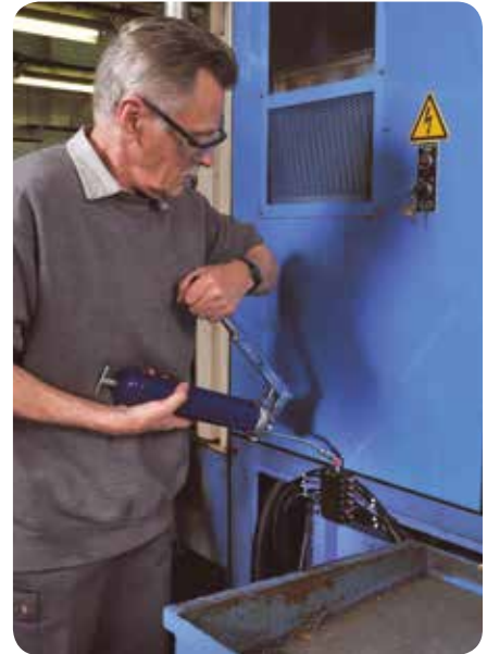
This single-point metering valve enables this technician to lubricate ten bearings without removing any guards or shutting down the production line.
