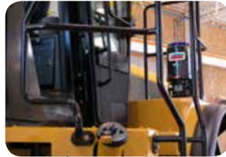
Customized pump mounting for ease of monitoring and refilling
