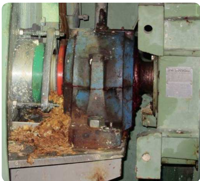
Fig. 6 Fibre leaking out of the gland seal on a pulp washer. Note the additional protection in front of the housing to protect the housing seal.
