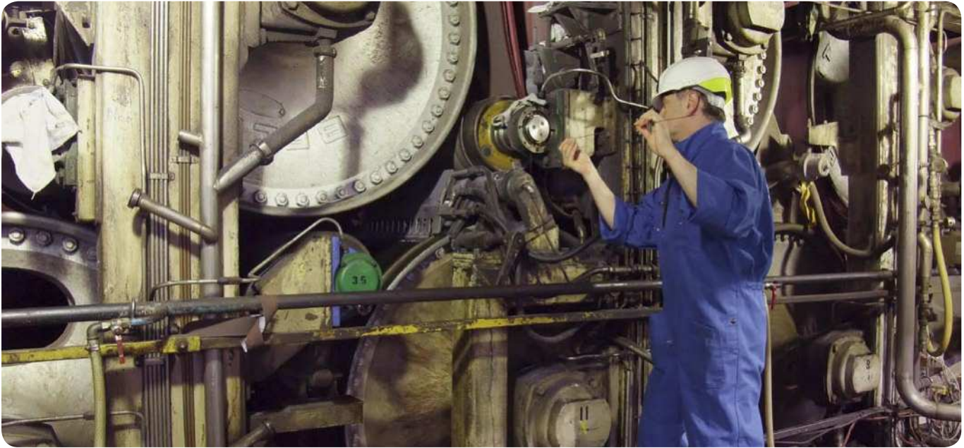
Philippe Gachet using a wire tool to check the condition of the raceway on a felt roll bearing.
