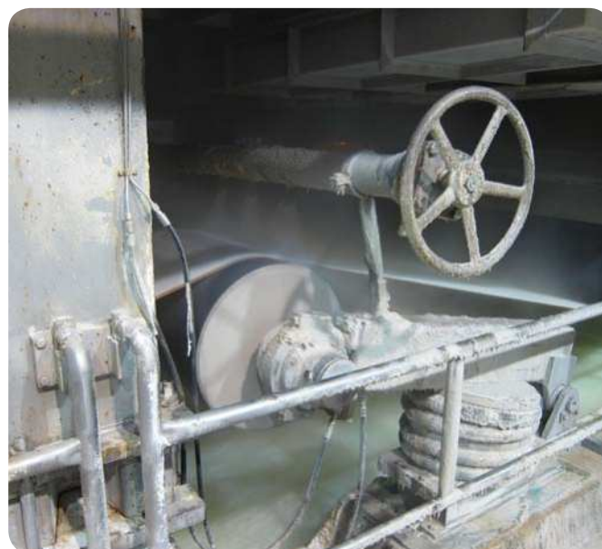
Fig. 7 The high humidity environment of a wire stretch roll in a paper machine forming section. Grease in the labyrinth seal stops process water entering the bearing housing.
