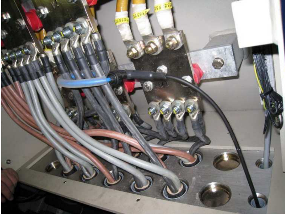
Figure 3 - 7. Flexible Load Sensor Measuring One of the Generator Phase Cables.
