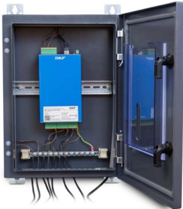
Figure 3 An IMx device DIN rail mounted in IP65 cabinet
