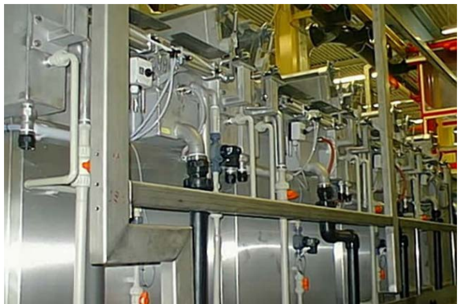
Phosphating plant at SKF
