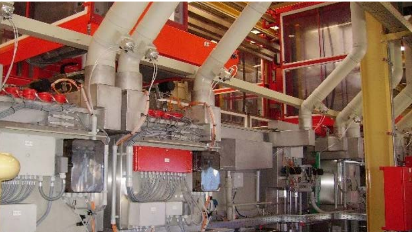
Chemical treatment plant at SKF
