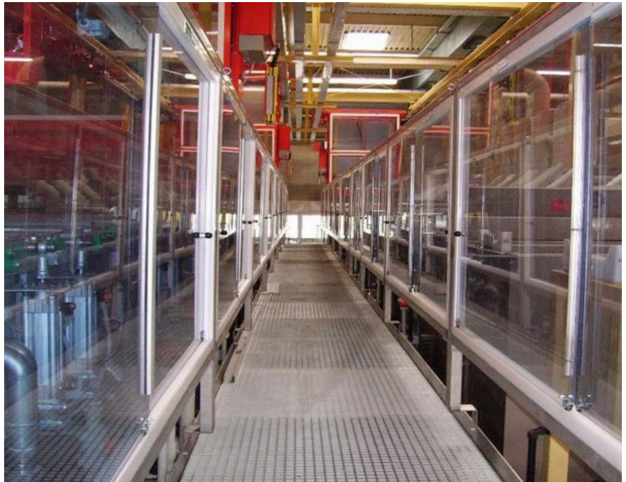
Coating plant at SKF Schweinfurt, Germany
