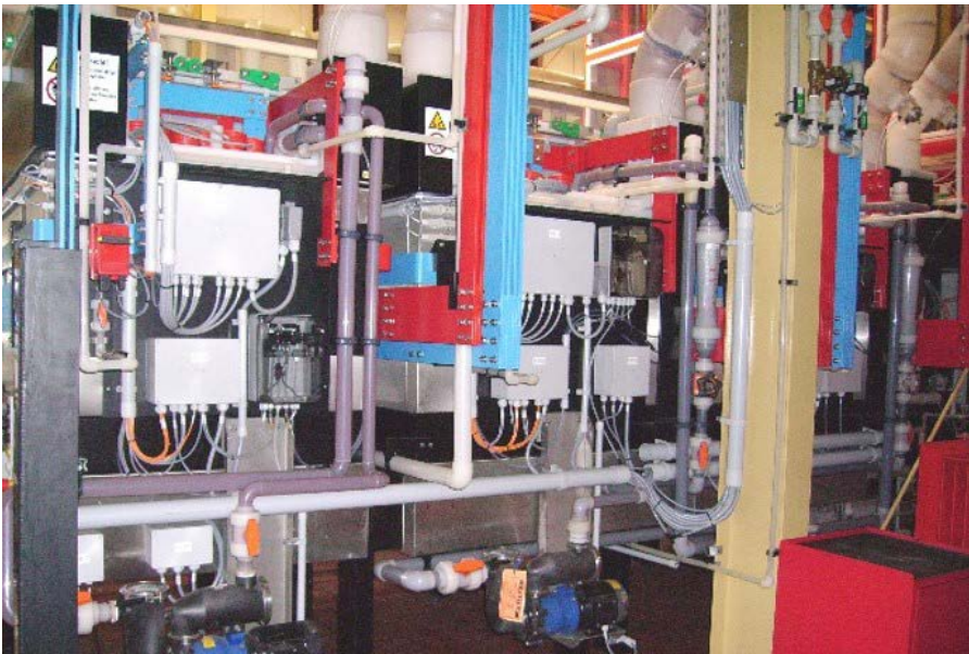
Galvanic coating plant at SKF
