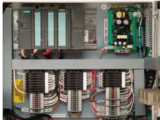
Fig. 05 Programmable Logic Controller (PLC) and Electronics
