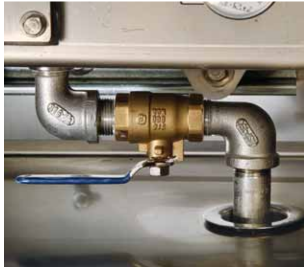
Fig. 19 Reservoir Drain Valve and Enclosure Drain Port
