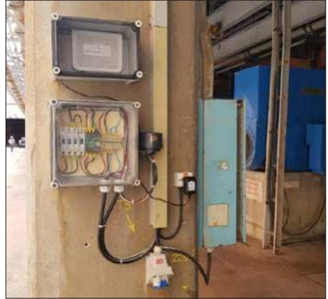
Fig. 1 – Select a clear area with good GSM signal. The concrete pillar could block all signals. Ideal place for the gateway is high inside the building without wall interferences.
