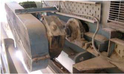
Split block in a trapped position.
