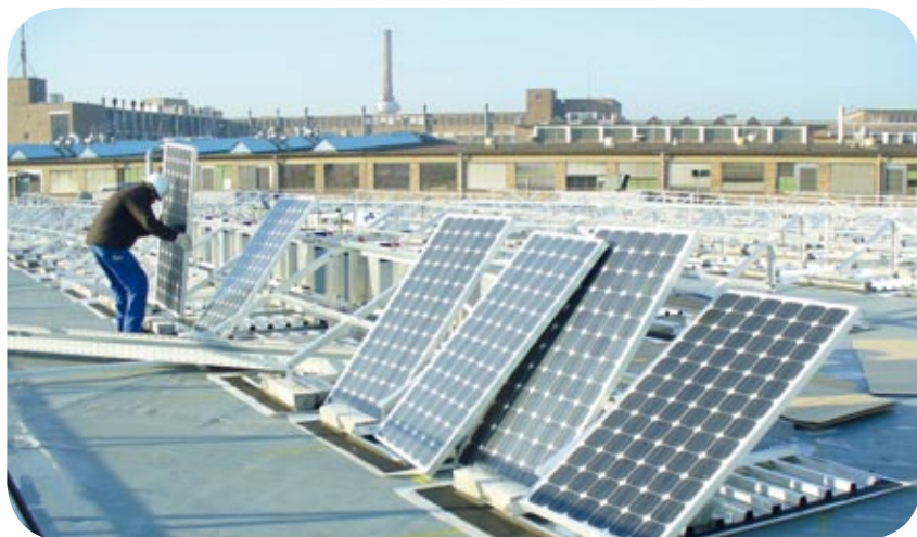
SKF Logistics Services Centre in Schweinfurt, Germany invested in a major solar panel project, covering its 15,000m 2 roof structure.
